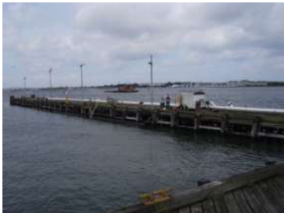
Cape May Deteriorated Pier
