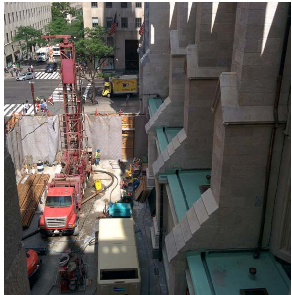
St. Patrick's Cathedral Geothermal Heating & Cooling System P.W. Grosser Consulting Landmark Facilities Group, Inc.
