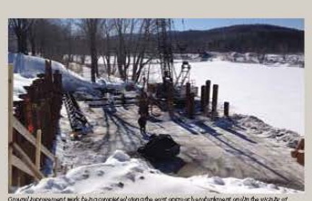
Ground improvement work being completed along the west approach embankment in the vicinity of Abutment 2.
