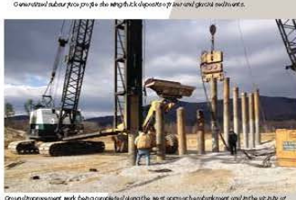
Ground improvement work being completed along the west approach embankment and in the vicinity of Abutment 1.
